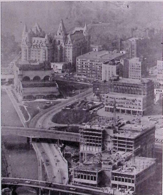
NEW CFHQ GROWS UP - Located between the Laurier Avenue and MacKenzie King bridges adjacent to the east bank of the Rideau Canal is the new Canadian Forces Headquarters building in the foreground. Construction crews are now pouring concrete at the ninth floor of the twin-tower, 20 storey building. In the background is the Chateau Laurier Hotel rising above the Ottawa River. (Canadian Forces Photo)
