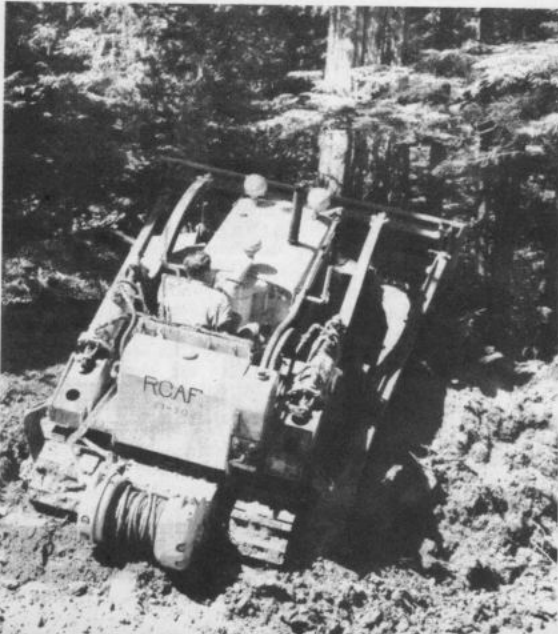
Cats climb trees — almost. Sgt. G. Downs of Milton, Ont., bucks his bulldozer against a cedar, chunking out muck and timber in bush station's private war against nature.
