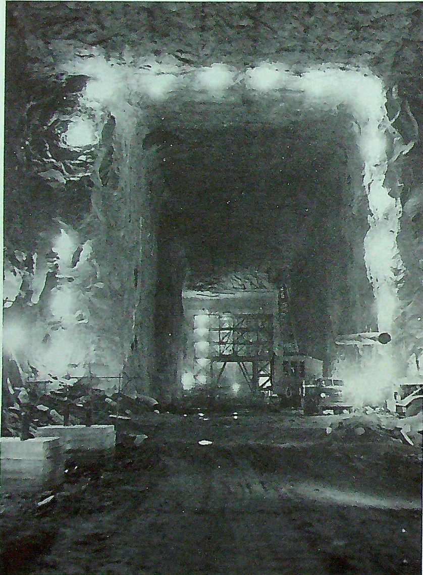
A gantry crane in one of the main chambers.
