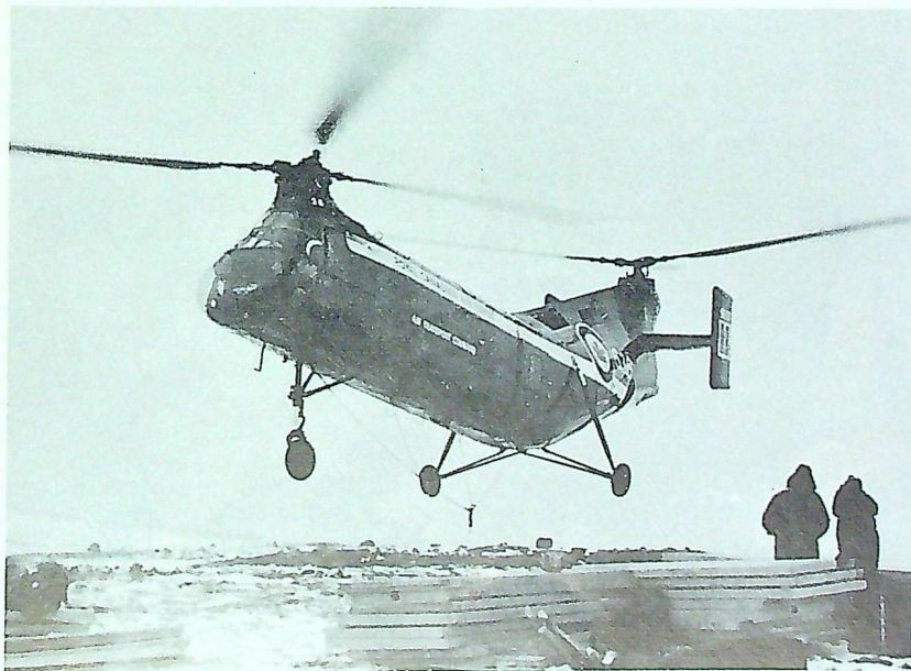
Vertol H-21 heads back to marshalling area after depositing load at MCL construction site.
