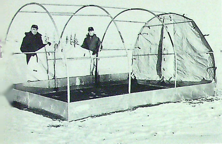
A Janesway hut being erected by R.C.A.F. personnel during a joint Army/R.C.A.F. exercise.
