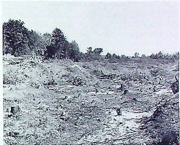
Clearing the ground for the construction of runways at No. 10 E.F.T.S., Pendleton, Ontario.
