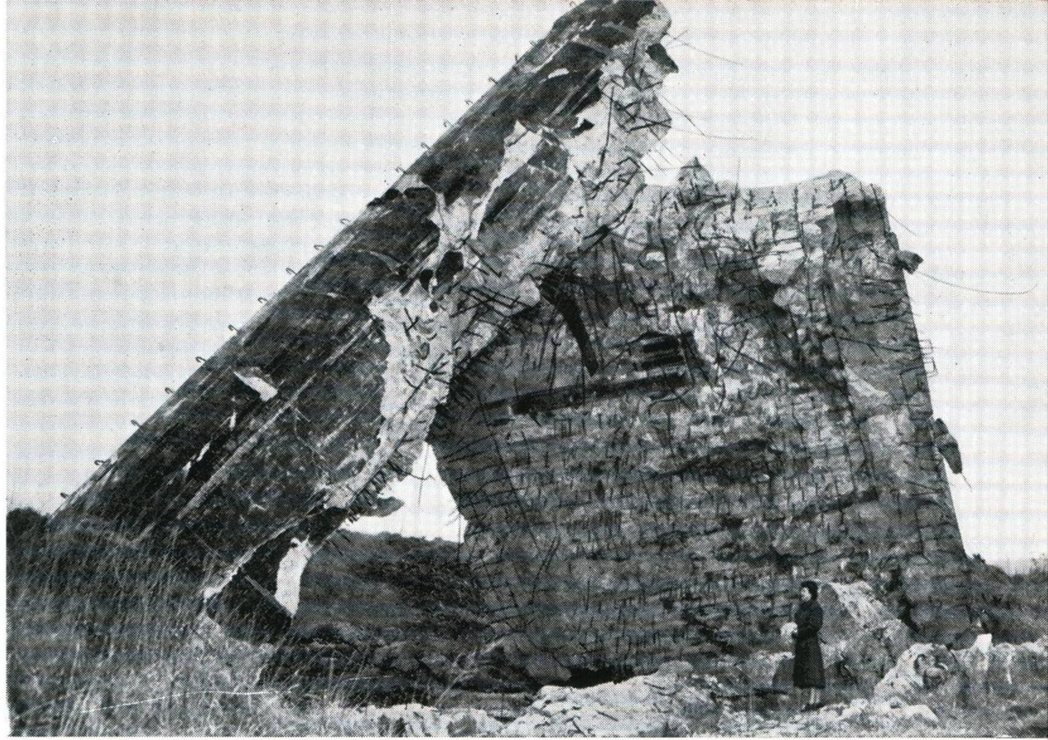
Some idea of the size of this demolished bunker can be gauged from the airwoman standing in the bottom right hand corner of the photograph. It stands in the middle of a farmer's field, a few hundred yards from the airfield boundary fence.
