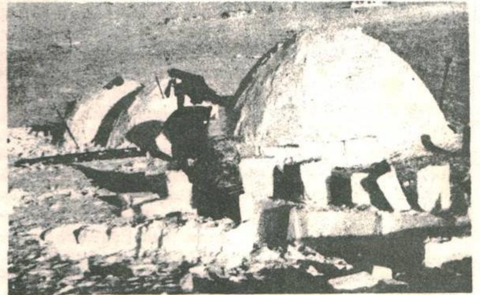
These men building igloos could be either Eskimos or Royal Canadian Mounted Police setting up new quarters. Both have at least two things in common; they are adept at building snow houses and are concerned about air defense. All support the GObC.
