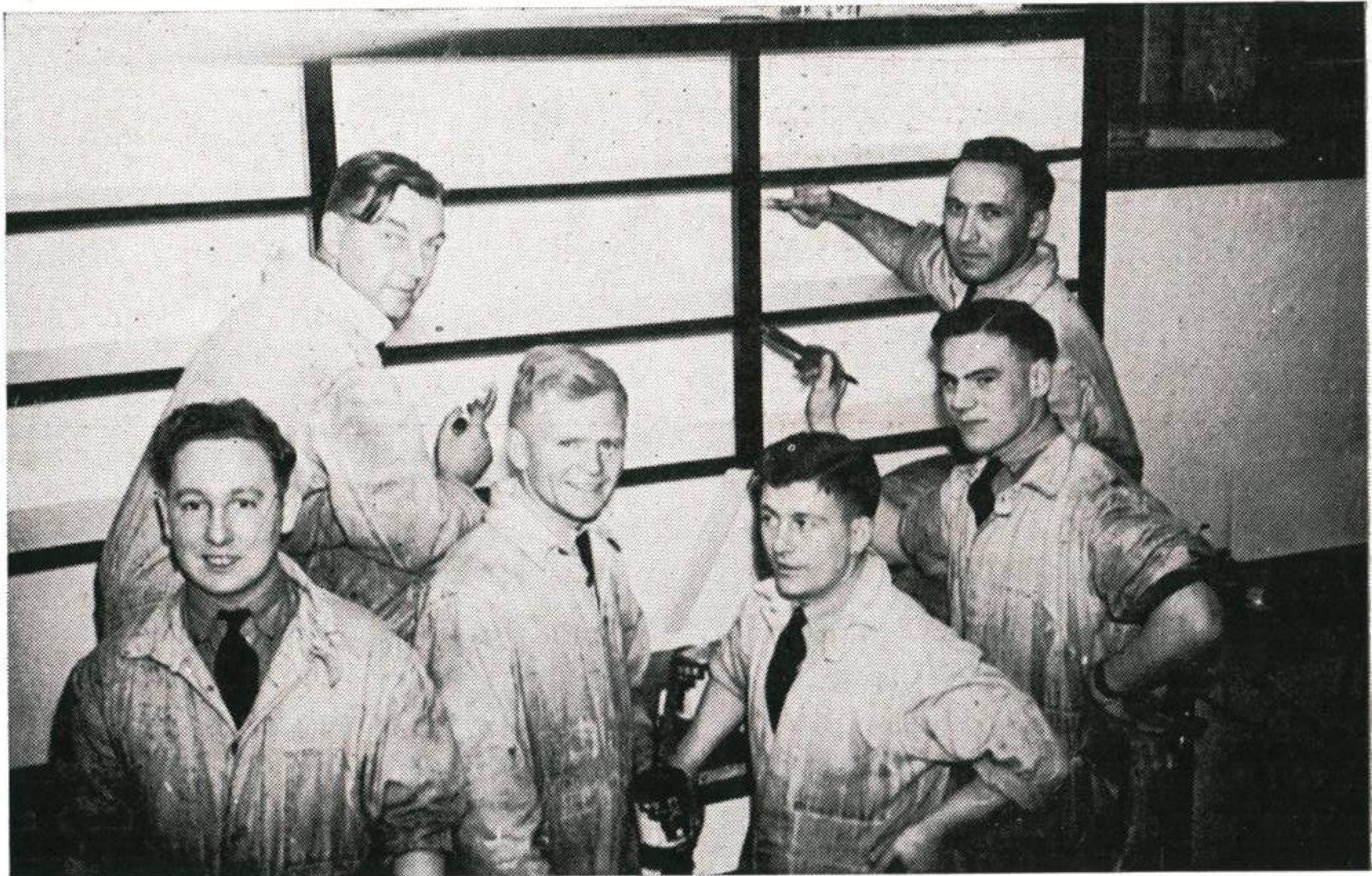
Here's the "Painter Patrol" giving the final touches to the Station Cafeteria. In the usual order: AC. Leach, AC. Hermon, AC. Wilson, LAC. Gotts, AC. Hukin, AC. Taylor (LAC. Sherington is missing from this photograph.)
