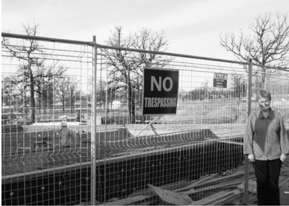
Assistant Director of the MFRC Child Care Centre, Cathy McCullough shows off the progress being made on the expansion of the daycare centre that will allow them to offer more temporary infant care spaces to military families being posted to 17 Wing Winnipeg. Photo: Alison Dickey
