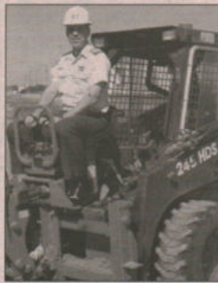
Col Kummel initiates demolition of an obsolete Det Dundurn building while visiting the Detachment.
