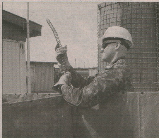
Master Corporal Francois Cross, a member of 1 Combat Engineer Regiment serving with the 2 PPCLI Battle Group in Bosnia connects two Hesco Bastion units together using a spring. The retaining walls are being used to build new bunkers at Camp Black Bear, Velika Kladusa.
