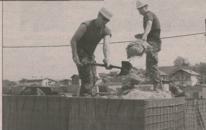
Corporals Danny McKluskie and Mike Scoretz, members of 13 Field Squadron, 1 Combat Engineer Regiment serving with the 2PPCLI Battle Group, level off the Hesco Bastion retaining walls. The retaining walls are being used to build new bunkers at Camp Black Bear, Velika Kladusa in April 2003.
