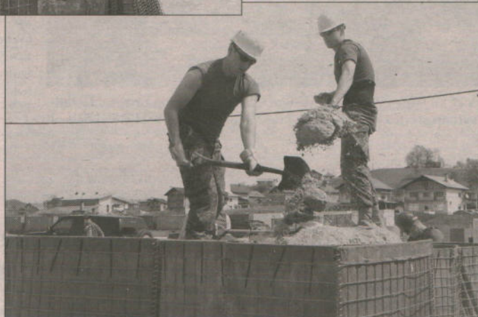
Corporals Danny McKluskie and Mike Scoretz, members of 13 Field Squadron, 1 Combat Engineer Regiment serving with the 2PPCLI Battle Group, level off the Hesco Bastion retaining walls. The retaining walls are being used to build new bunkers at Camp Black Bear, Velika Kladusa in April 2003.
