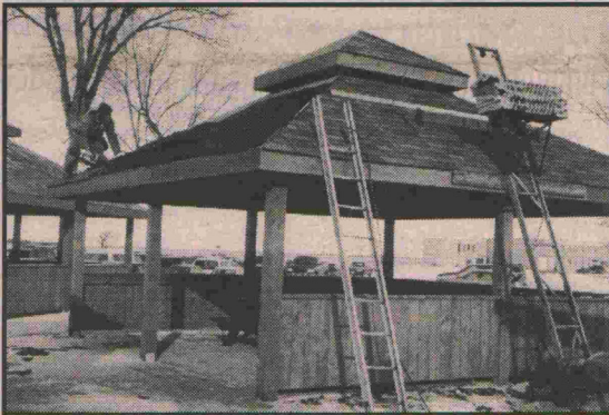
Snow may have fallen, but the patio is in and finishing touches are being made (Dec 99).
