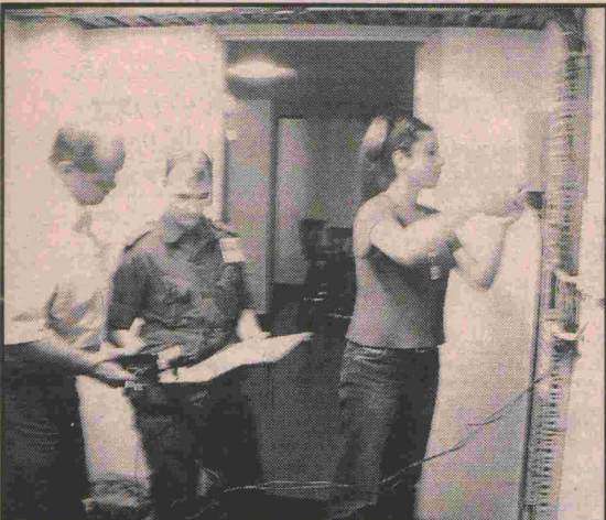
Ms. Adria Trumble and Cpl James Clarke from WTIS work with an MTS technician installing extra phone lines in Building 61. One third of the new lines are going into the Jr. Ranks Mess, the new location of several organizational sub-groups working for the Pan American Games. MTS and W TIS are adding two data circuits, 11 payphones, and 138 extra phone lines overall, in preparation for the Athlete's Village.
