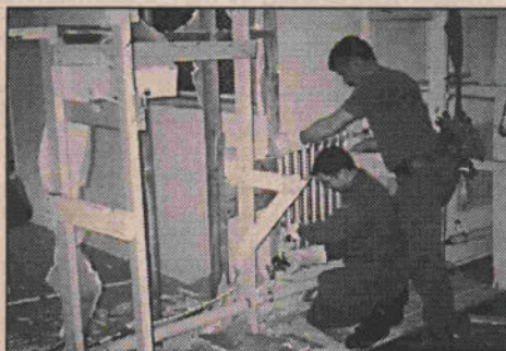
MCpl Steckly and Cpl Fortin during a removal of cast iron radiators from the steam heating system.
