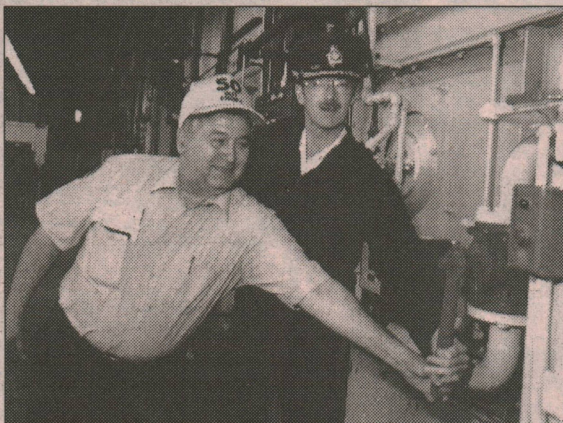
Seen here are LCol Smith and Mr Ed Myslicki "closing the gas valve" thus ending the production of high pressure steam at Bldg P5(S).
