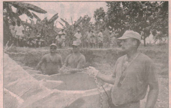
Left to right) Sergeant Lloyd Larsen, from CFB Cold Lake; Corporal Ted Boutin, from CFB Winnipeg; and Master Corporal Ken Purcell, from CFB Greenwood, and all members of the engineer battalion, are working on a humanitarian project of saving erosion of fertile soil.
