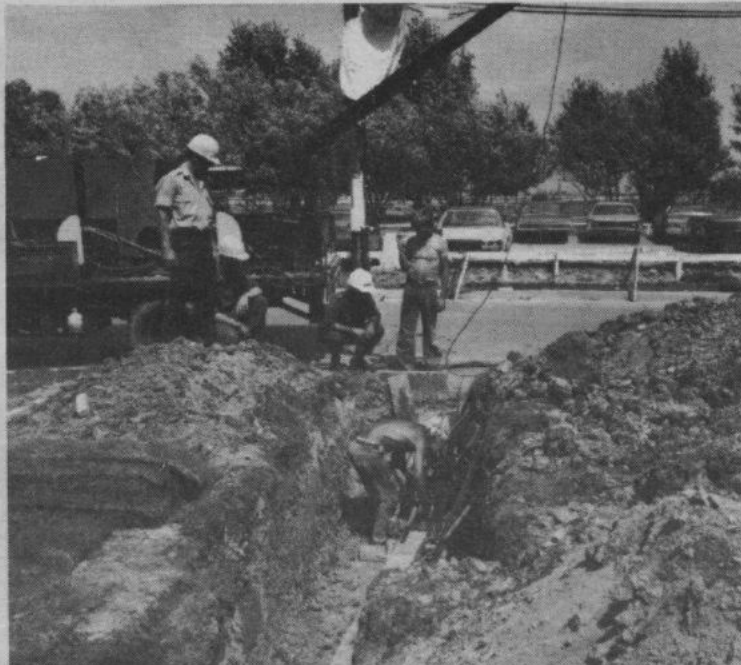
MCPL Terry Fuller (Head gopher) supervising laying of new telephone cable under road in front of HQ Bldg 87 CFB Winnipeg. (BASE PHOTO)
