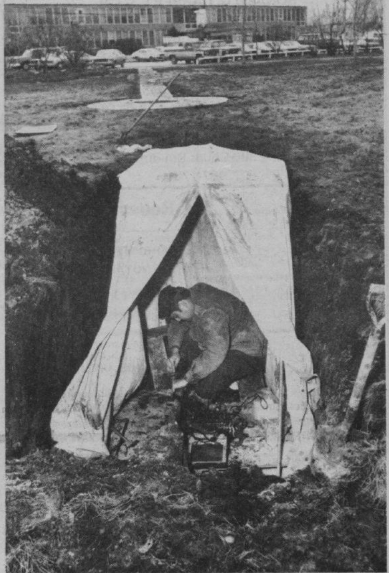
MCPL Eric Taylor (Lineman for the County) making repairs to cable. (BASE PHOTO)
