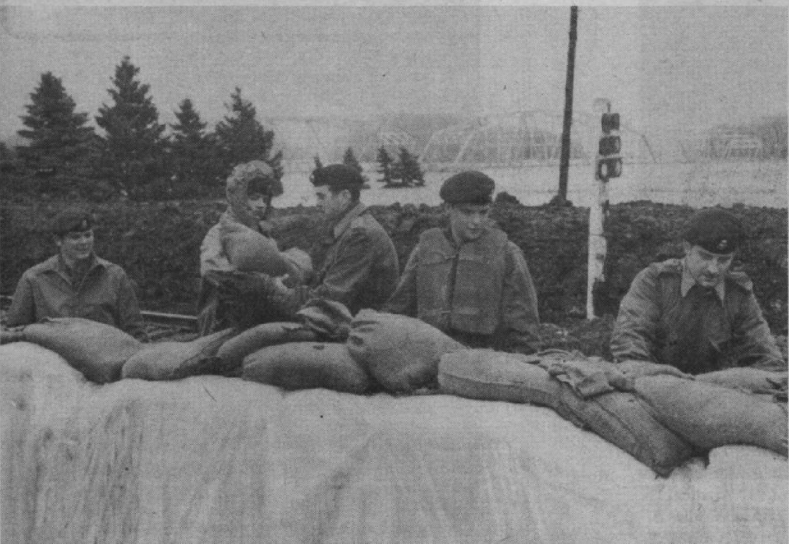
A "ring dike" at St. Jean Baptiste is built to prevent further leakage. (CF PHOTO BY WO J. CASEY)
