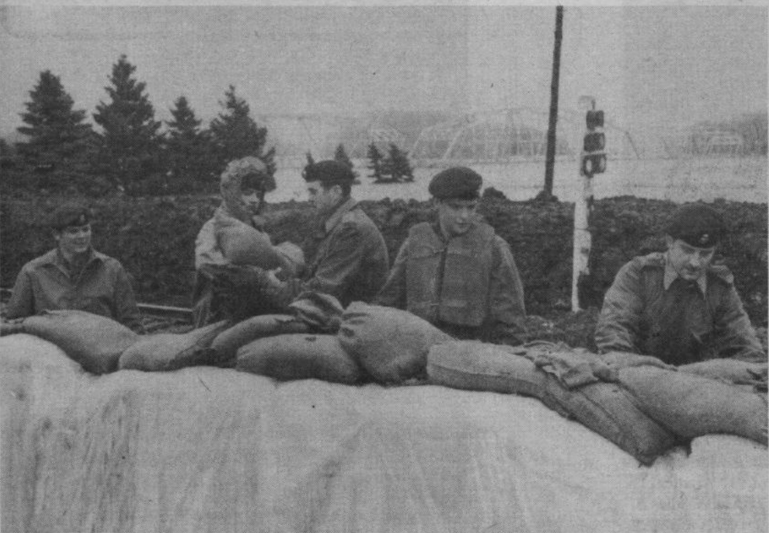
A "ring dike" at St. Jean Baptiste is built to prevent further leakage. (CF PHOTO BY WO J. CASEY)
