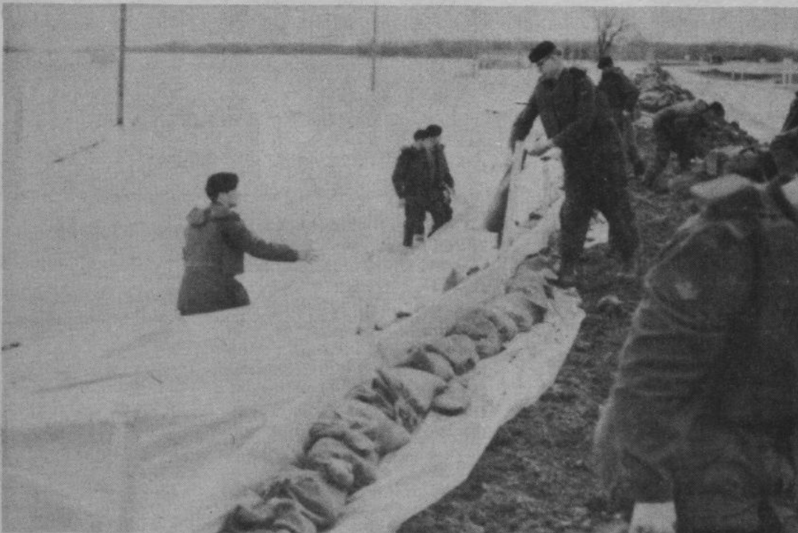
Protective sheeting is "anchored" to a dike using sandbags as weights. (PHOTO BY CAPT J. CASEY)
