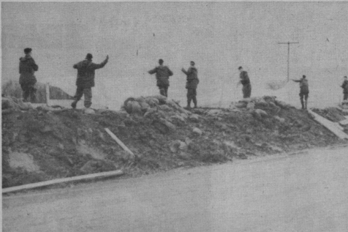
Troops of 2PPCLI lay protective sheeting over a dike to prevent erosion.(PHOTO BY CAPT J. CASEY)
