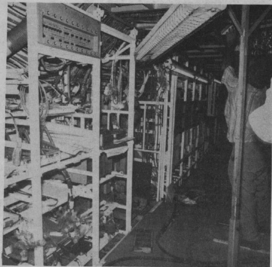
One week later, the equipment racks, less their covering doors, stand waiting the installation of the avionics black boxes. The large opening in the middle of these racks awaits the largest and most important of them all the General Purpose Digital Computer, the heart of the CP-140. (BASE PHOTO)
