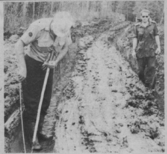
CAPT. Currie and MWO. Doyle of the CE Section assess the work to be done on the entrance road. (BASE PHOTO)
