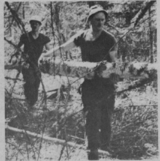
Site clearance required a lot of muscle power. SGT. Mullen manhandles a log while LT. Pelletier looks for the next victim. (BASE PHOTO)
