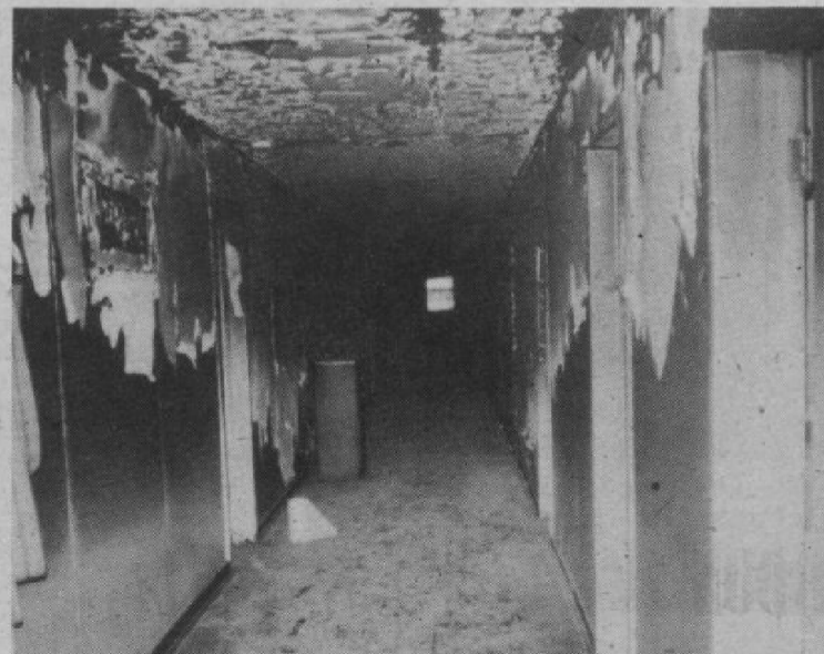
Within seconds, flames travelled the entire length of the second floor hallway.
