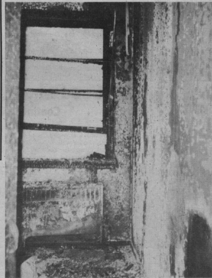
The fire started in this end room.
