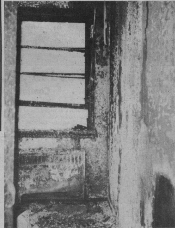
The fire started in this end room.
