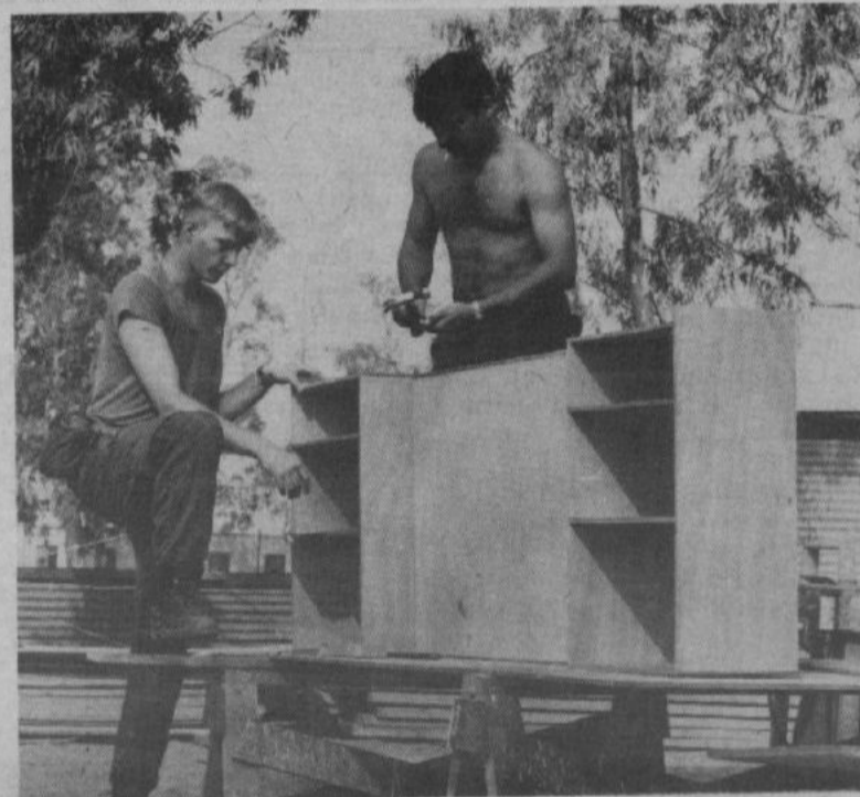
Newly constructed shelves are a welcome addition to local buildings in Ismailia, Egypt, as they are assembled by Canadian servicemen Master Corporal R.G. Kapusta, 25, formerly from Canadian Forces Base Moose Jaw, and Private R.W. McNaughton, 21, formerly of CFB Winnipeg. Both men are now stationed with the Canadian contingent, United Nations Emergency Force, Middle East. Cpl. Kapusta is the son of Mr. Val Kapusta, 3276 East 7th Street, Vancouver. Pte McNaughton is the son of Robert McNaughton, 1607 5th Ave., Grand Mere, P.Q.
