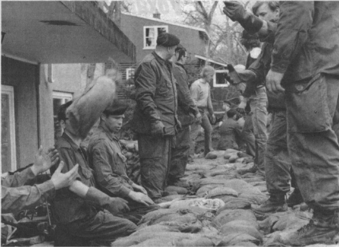
Military personnel worked around the clock shifts building ring dikes to protect homes. Diking operations were completed well in advance of the Red River reaching its crest. Base Photo
