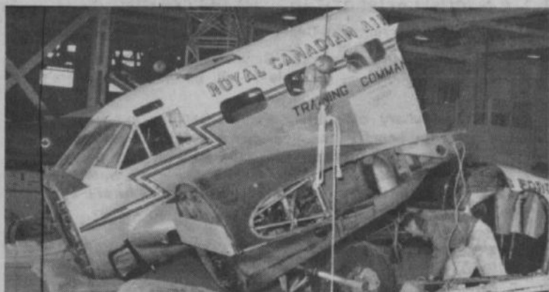
12 March Now to rotate this section 90 degrees. Sgt Ron Swayze ensures that the tires is clear as the section is raised
