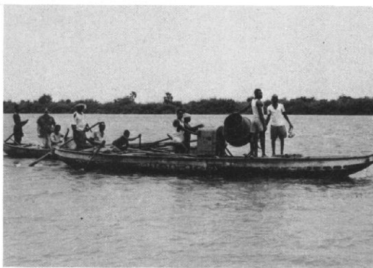
THE CEMENT MIXER, one of the few mechanical aids used in school construction, is moved across the Volta to the construction site.
