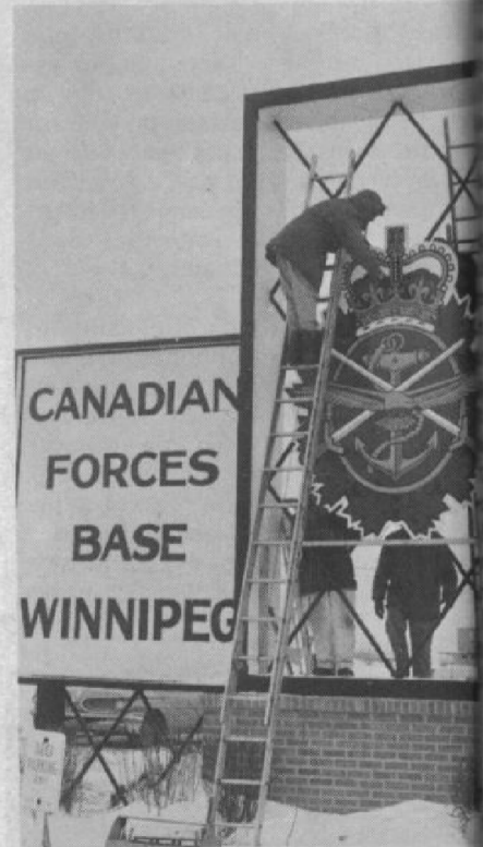
Workmen erect the Canadian Forces emblem at CFB Winnipeg, Thursday, Feb. 1, the day on which the Canadian Forces Re-organization Act was proclaimed. (Canadian Forces Photo)
