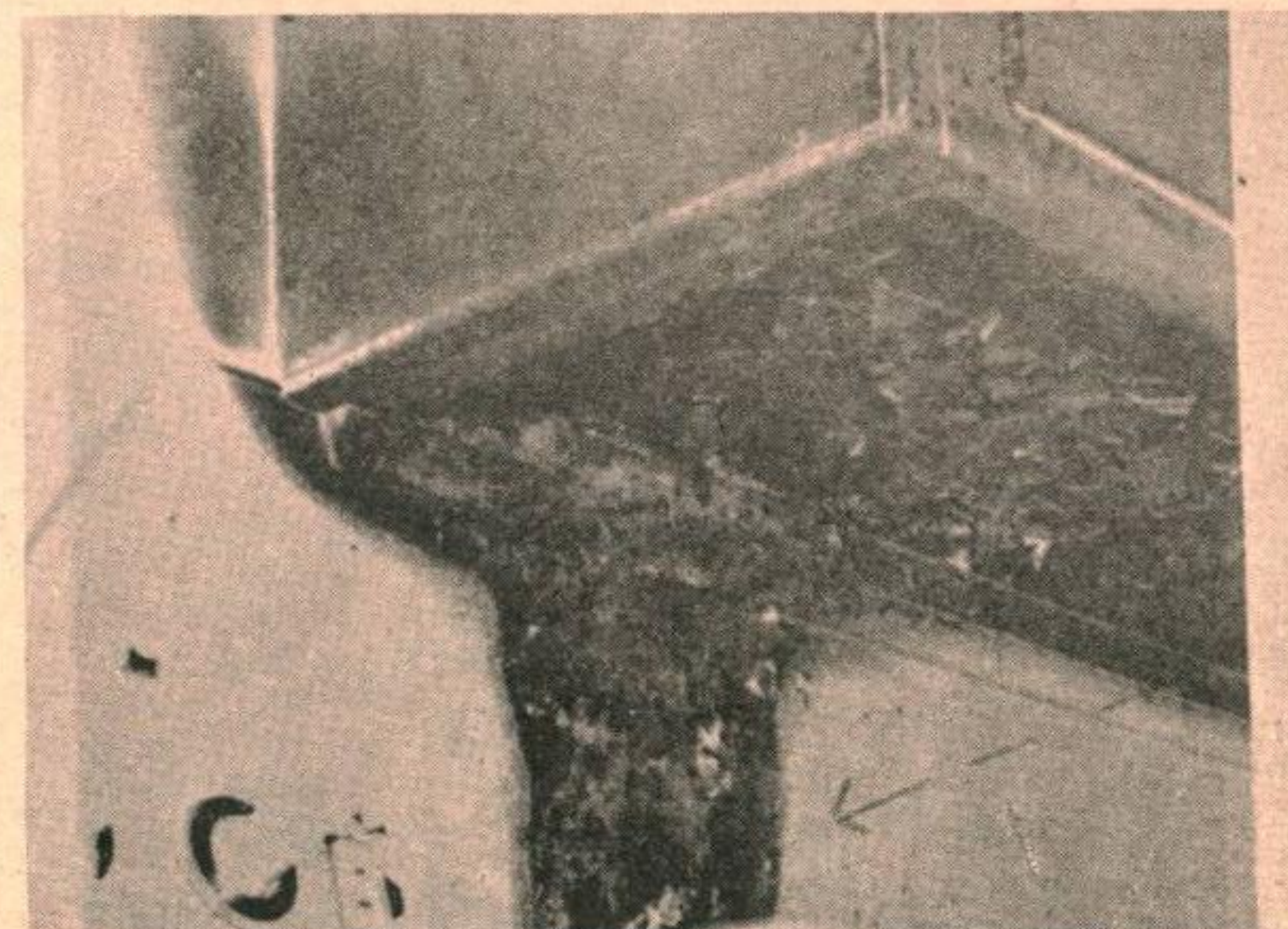
Heat radiated from a toaster to cloth pot holder hanging on the wall.
